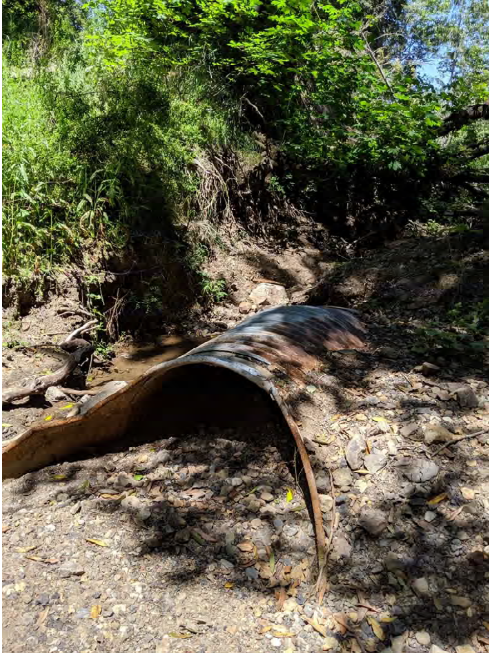
Photo 3. Delineated other Waters at Data Point P01, looking west to east across study area corridor, showing damaged, non-functional culvert in stream channel.
